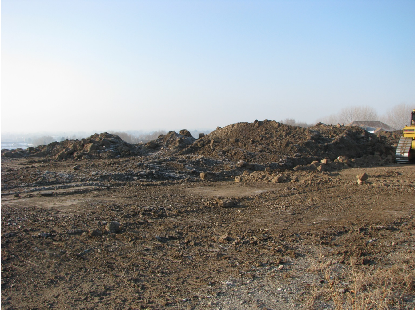
Looking southwest at the newly stock piles fill disposed of at the working face
